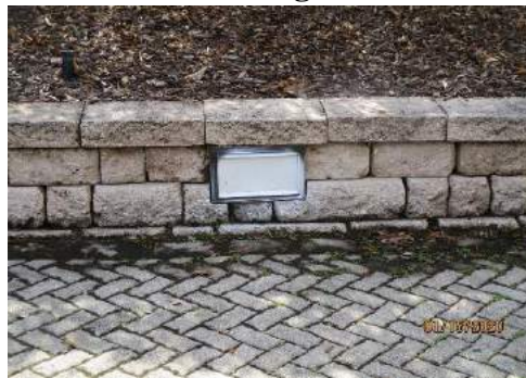
No Grate on Light Fixture
