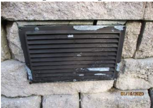
Peeling Paint on Light Grate
